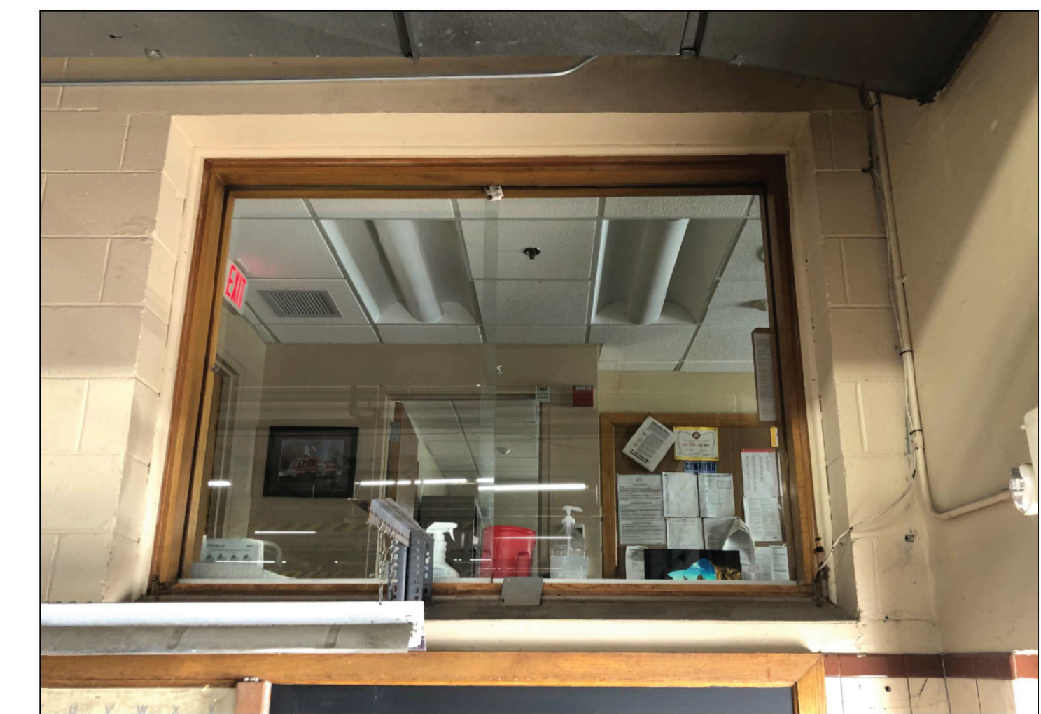
9 WINDCW - APPARATUS BAY SIDE
